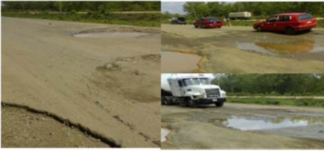
Figure 2. Failed Portion of Itobe-Ajaokuta Expressway.
