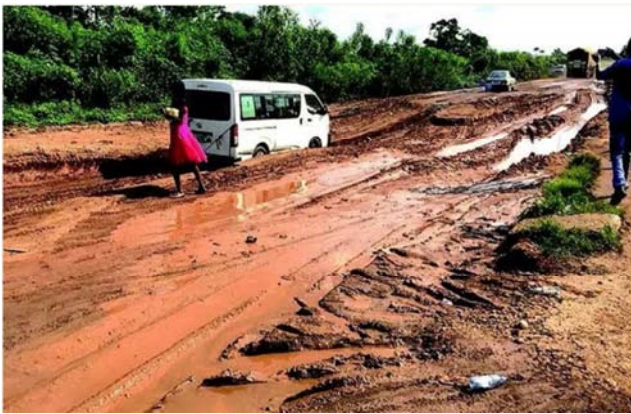
Figure 3. Failed portion of Itobe-Ajaokuta Expressway.
